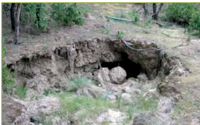
Figure 5. Piping failure or tunnel erosion in a dam constructed from soils derived from Permian mudstone. This dam is known to have failed on first filling. The image was taken from the dam floor.
