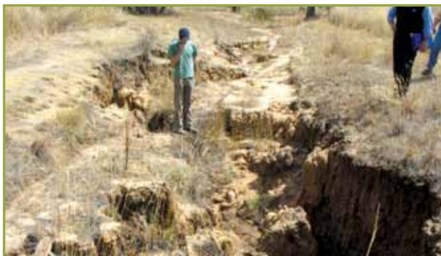
Figure 1. Tunnel and gully erosion resulting from construction of a stormwater culvert in dispersive clay.
