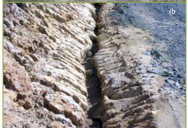
Figure 6 (a). Tunnel erosion resulting from construction of a culvert in dispersive clay (b). Tunnel erosion caused by installation of optical fibre cable in dispersive soil.
